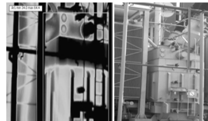
Gambar 4.5 Body Generator Transformer 1 (indonesia power, 2013)
